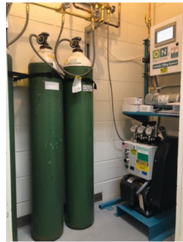
Oxygen cylinder filling station
