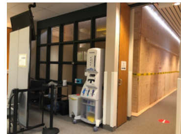
Skylight replacement: the hospital's main entrance with shoring and the swabbing station moved temporarily
